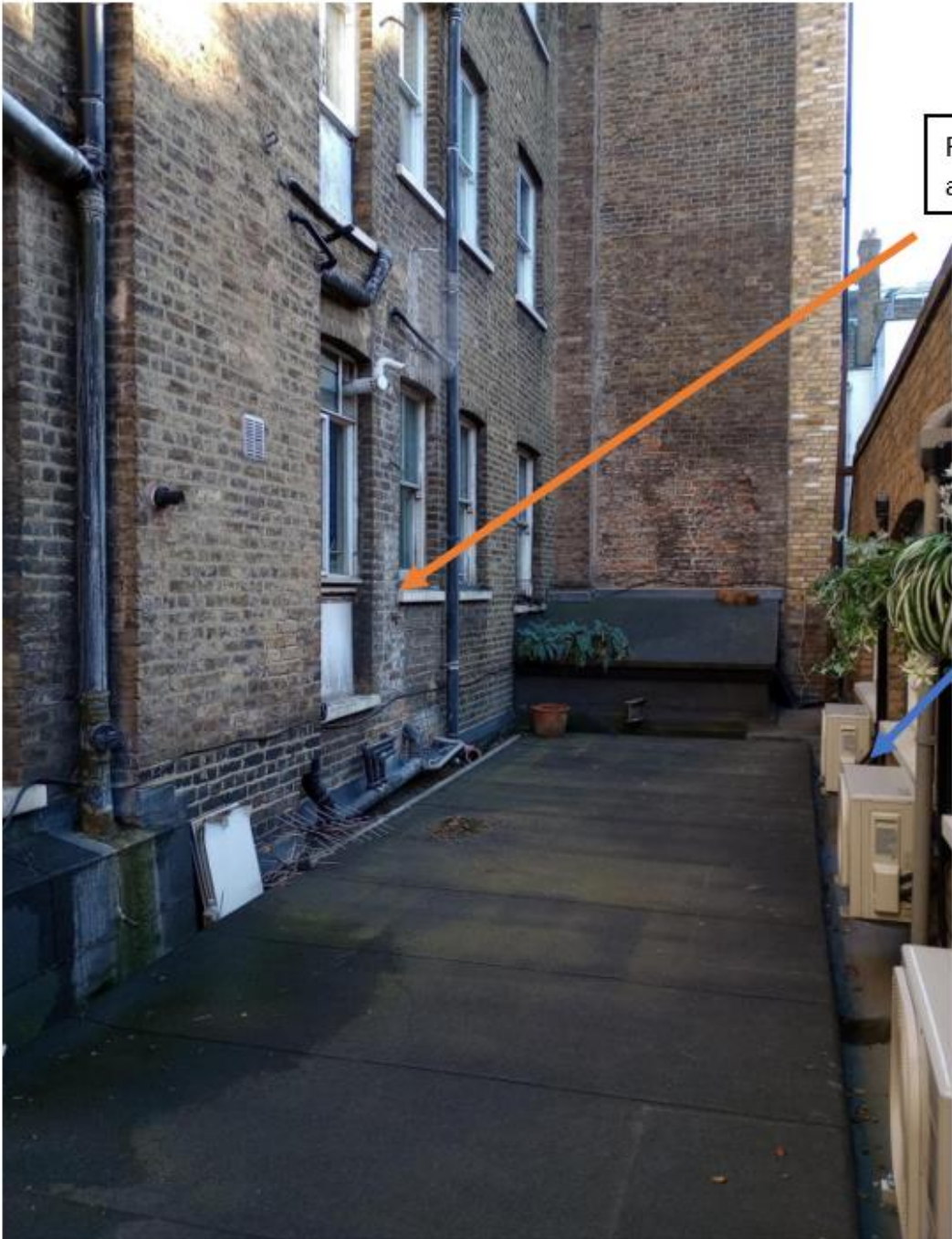
Photograph showing proximity of residential rear windows and plant equipment –
